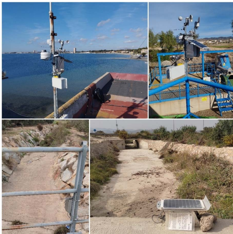
Fig. 7. Freestations installed in SMARTLAGOON project.
